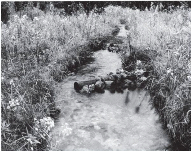
One task undertaken by each authority was the improvement of all streams in its watershed for fish life. Deflectors like these, often built with old barn beams and railway ties, create pockets of still water for trout. These examples were built on a tributary of the Saugeen.
